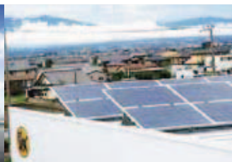
Solar power generation panels
